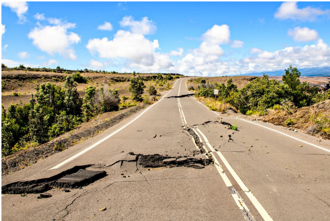
Earthquake causes major damage to roadway.
