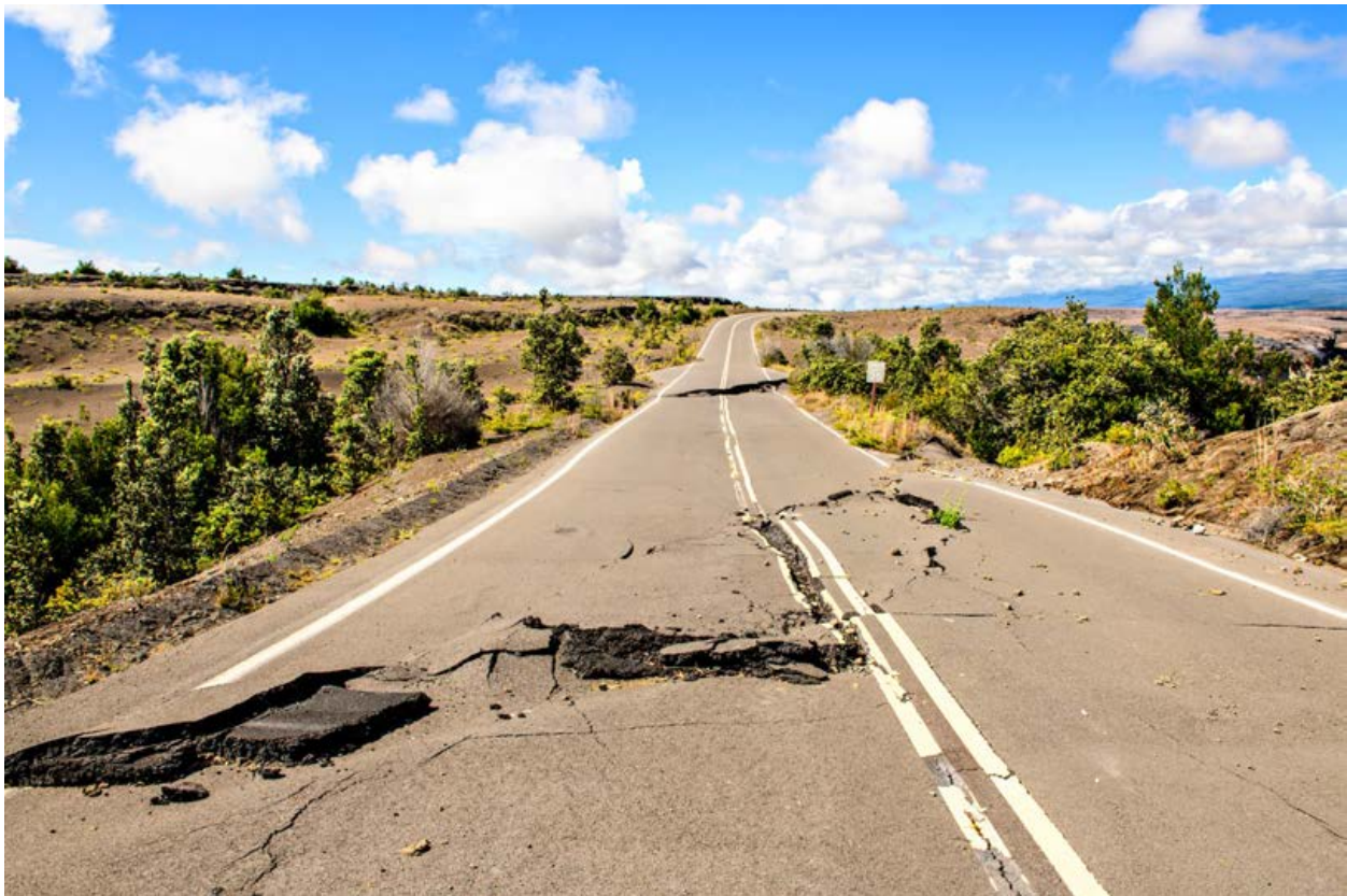
Earthquake causes major damage to roadway.
