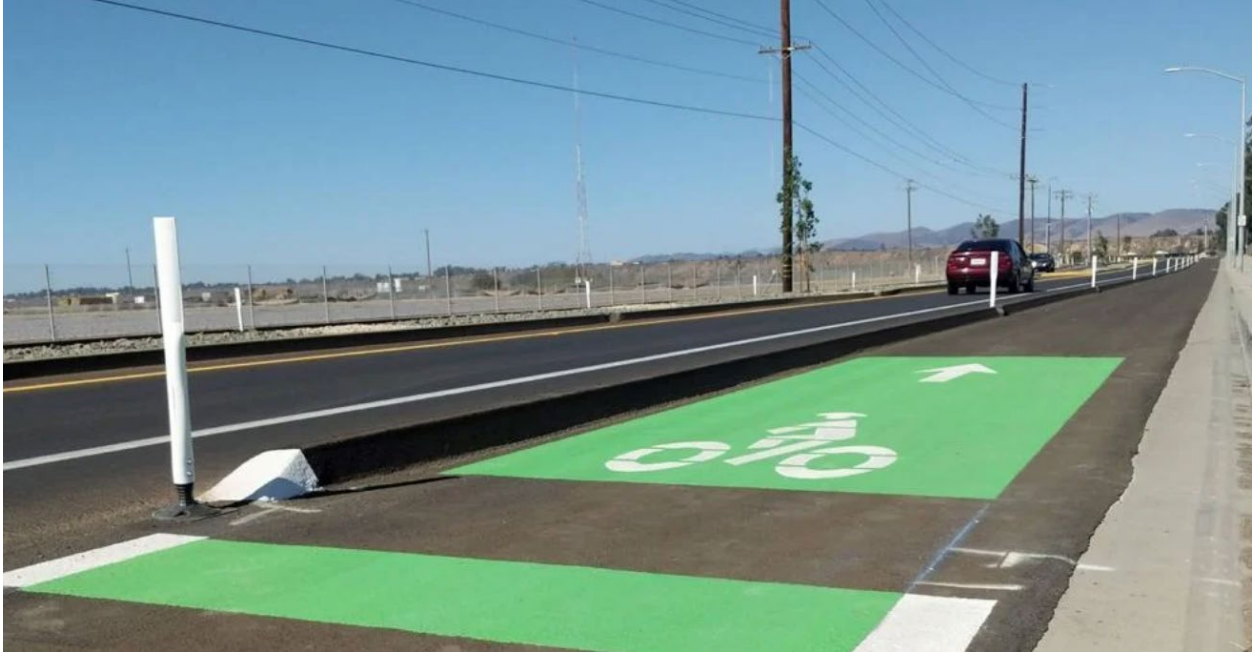
Protected bike lane installed on Blosser Road in 2023.
